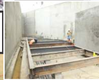
Chiller Platform, Netmagic Data Center - Bangalore
