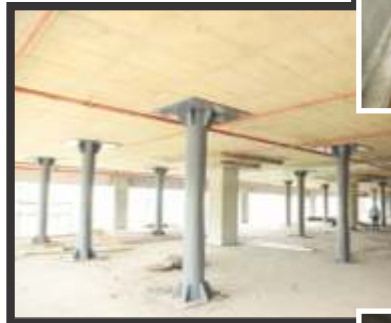
Circular Column Supporting - Tulip Data Center, Bangalore
